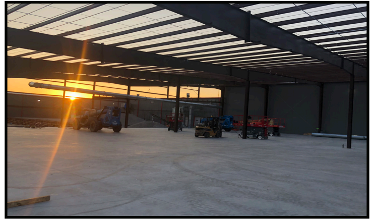
The steel skeleton at the Willow Springs, Missouri, facility, is being erected as the expansion project adds 35,000 square feet to the existing facility.
