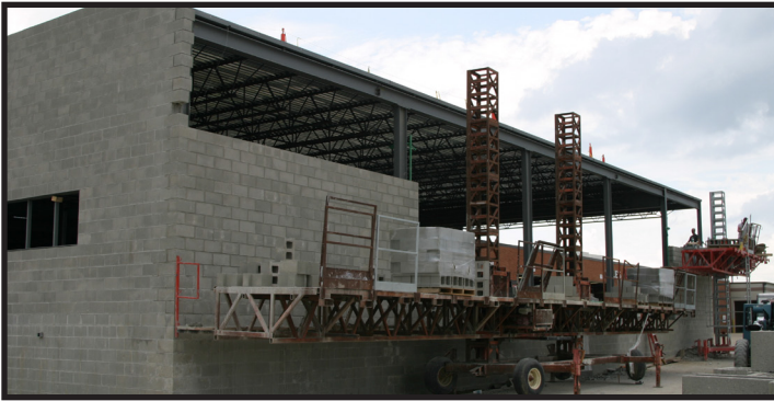
The Air and Fuel Components area is part of this 12,000 square foot Diesel Division expansion at JASPER's Wernsing Road facility.
