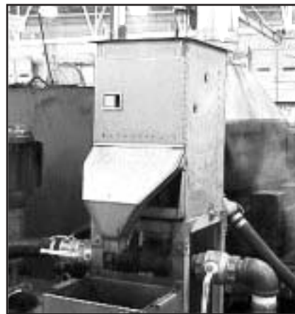
This filtration system at JASPER's Crawford County facility removes particles as small as 200 microns in diameter.
